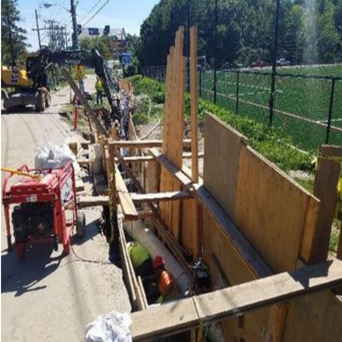
Fig 1: McCourt continues to install pipe in trench along Colovos Rd. Viewing south. (7-08-19).
