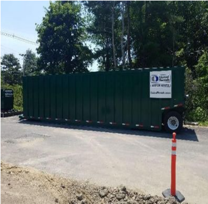
Fig 5: Frac tank for College Brook bypass. Viewing south. (7-09-19).
