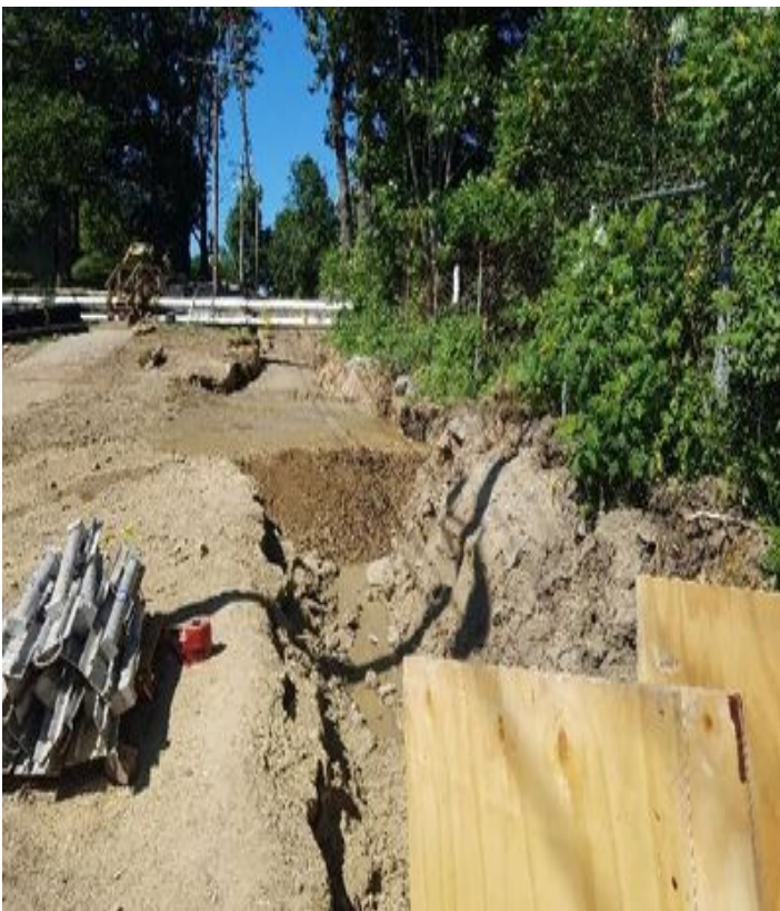
Fig 3: Concrete duct bank and float fill installed next to the field house cont. Viewing north. (7-08-19).
