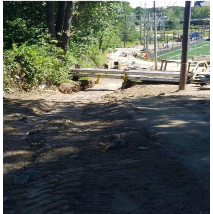
Fig 2: Concrete duct bank and float fill poured in trench next to field house. Viewing south. (7-08-19).
